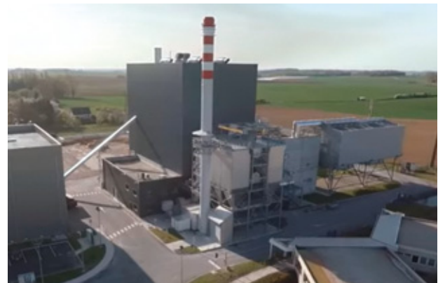
Biomass boiler recovering wood waste from a local forestry operation and supplying steam to the Bonduelle plant in Estrées-Mons (France).
